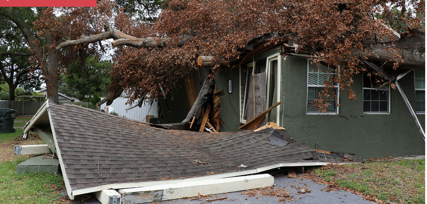
A Florida home damaged by Hurricane Irma in 2017
